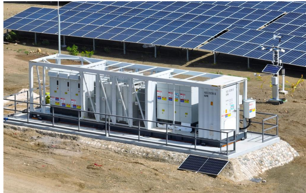
PI – INVERTER STATION
